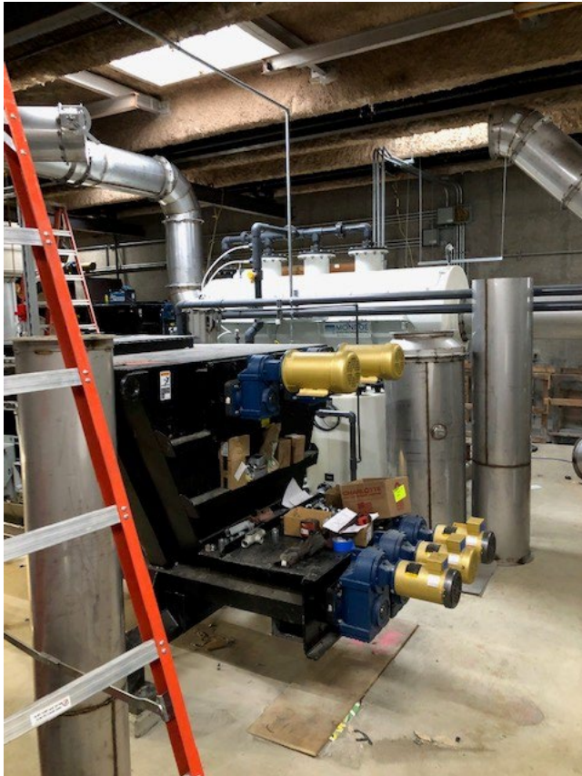
Packed Tower & Hopper in Upper level
