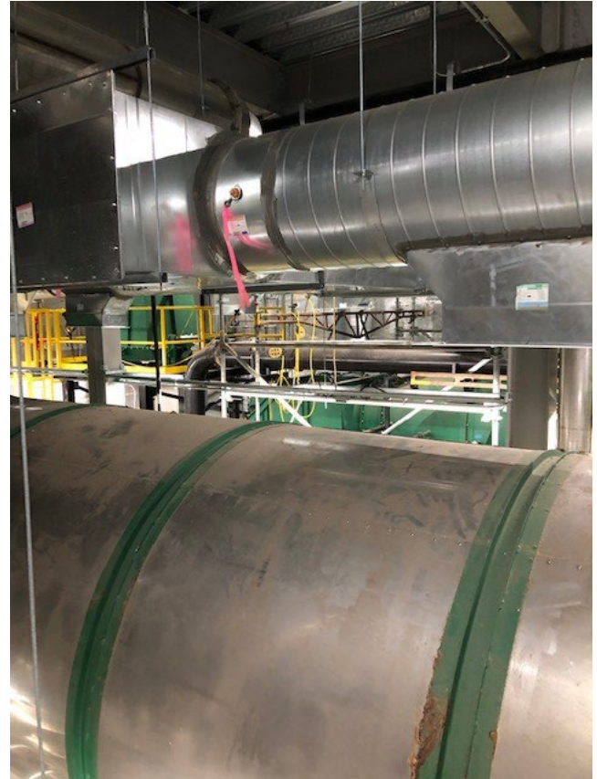
Gasification & HVAC Ducting in Lower level.
